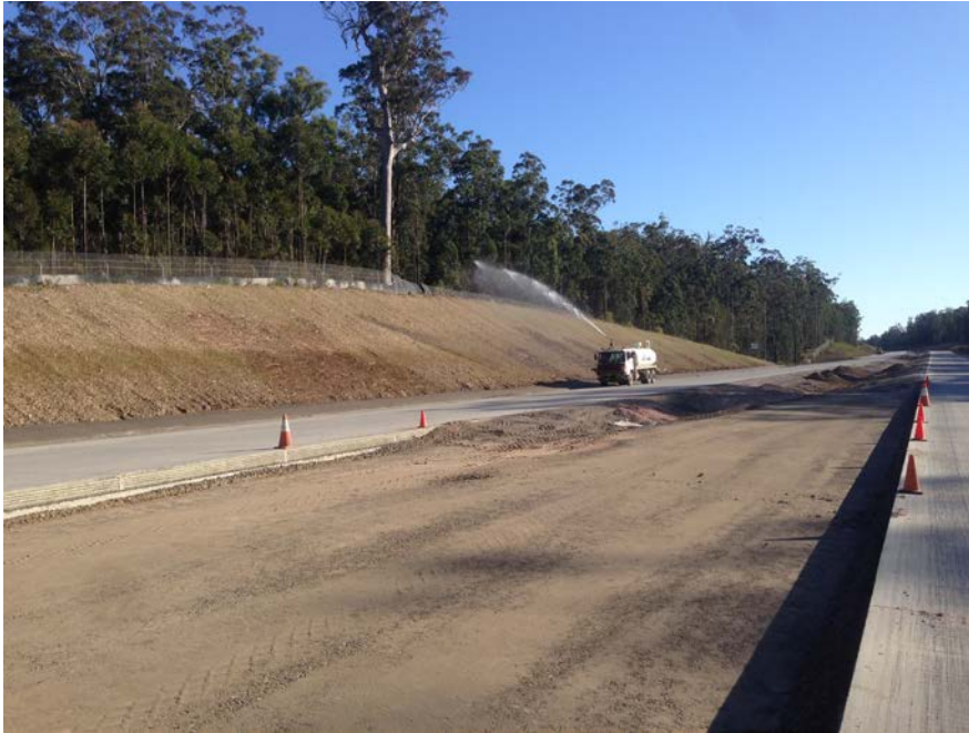
Watering of rehabilitated cut batters to assist in the establishment of cover crop
