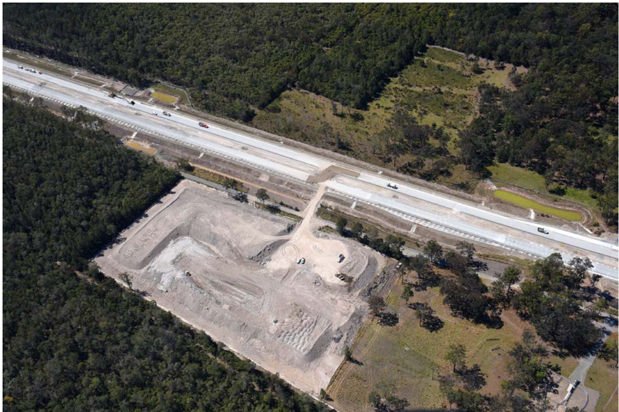
Ancillary facility for crushing surplus upper zone rock with rock and waste concrete
