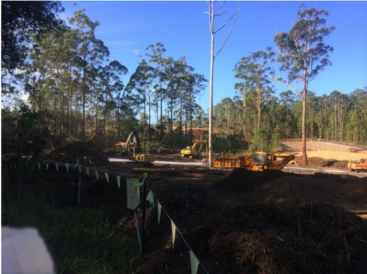
Plate 4: Example of a potentially hazardous HBT, in this case a stag, left within the work zone. Staff excavating drains and laying geofabric are within the fall zone of this tree.
