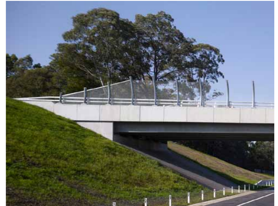
Typical Bonville Safety Screen termination
