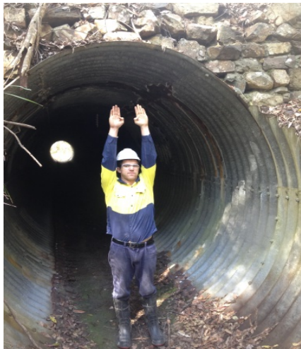
Plate 3. C599022 (chainage 22200) features 2x 3000mm galvanised pipes. The structure is likely a major microbat flyway and would present an entanglement hazard if curtained.
