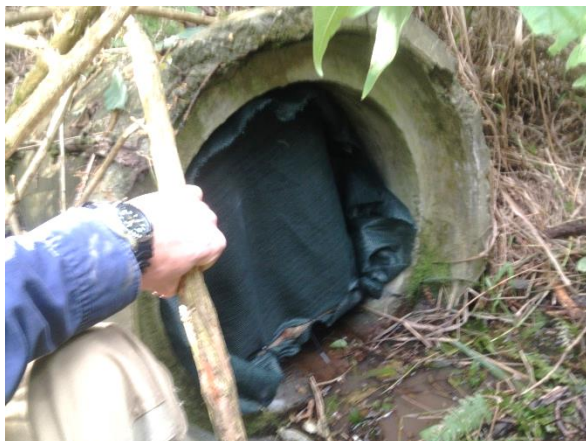
Plate 3. RCP 511067 (chainage 1000) was excluded with a nylon curtain after determining microbats were not roosting within the structure. The curtain features a 100mm gap at the base.
