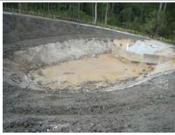
Permanent basin under construction with baffle boards and low flow pipe (St 2)
