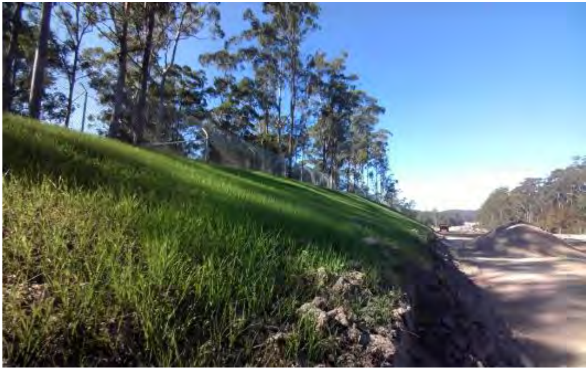
Permanent revegetation of the Cut 5 batter (St 2)
