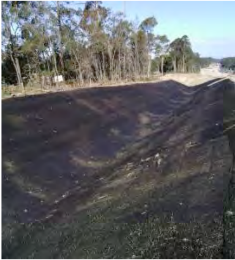
Permanent treatment of an open vegetated channel. This includes sub soil treatment, scarifying the subsoil, topsoiling, application of jute mesh, hydromulch and bitumen emulsion application (St 2)
