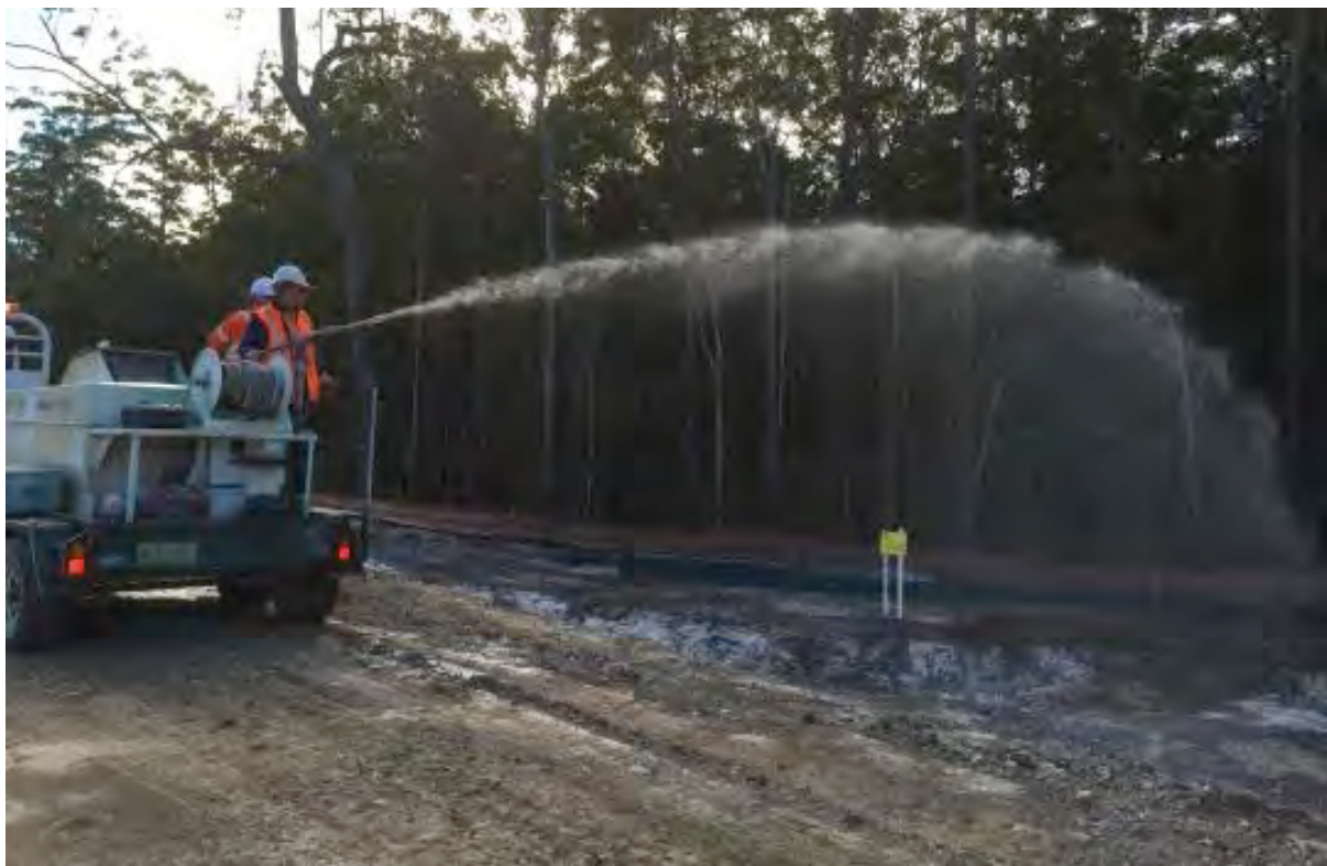
Application of gypsum and lime to the sub-soil pre topsoil application (St 2)
