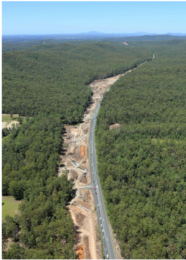
View south toward transition between Stage 2 and Stage 3 at Barrys Creek (St 2)
