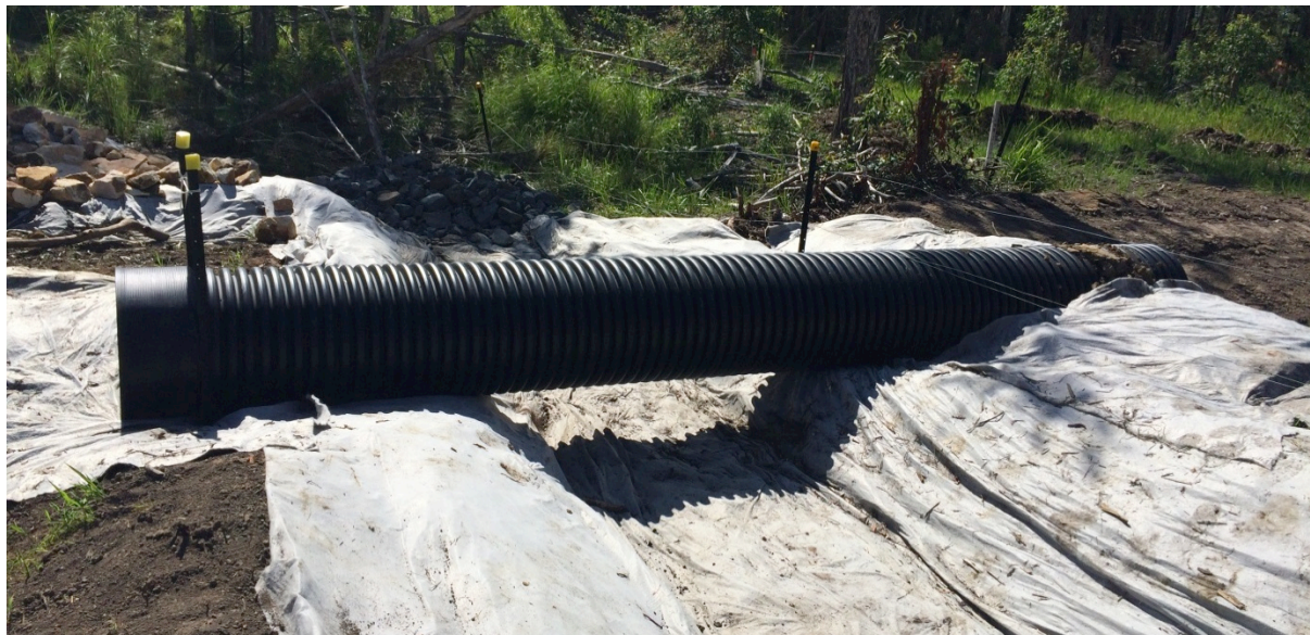
Construction water pipe - this pipe allows site water to flow to a licensed water quality basin without affecting a clean water diversion channel (St 3)
