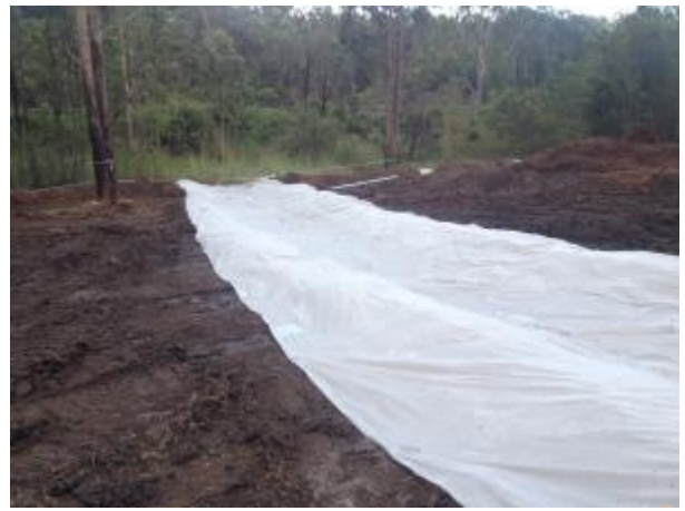
Clean water flow line (St 2)
