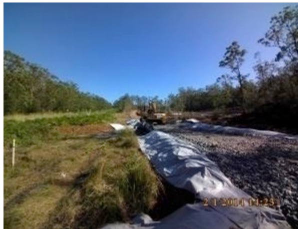
Clean water crossing (St 2)
