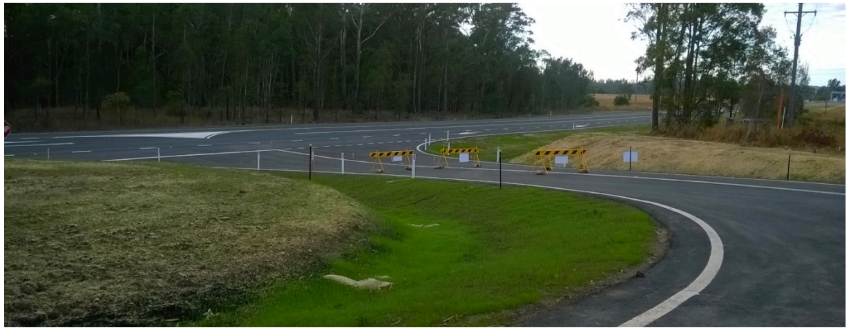
Revegetation of shoulders adjacent to Stage 3 contractor's site compound access and Ancillary Stockpile 3 (St 1).
