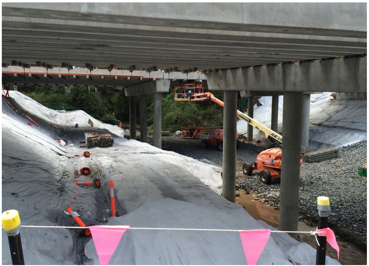
Pipers Creek October 2015 prior to removal of temporary low-flow pipe culvert (St 2)
