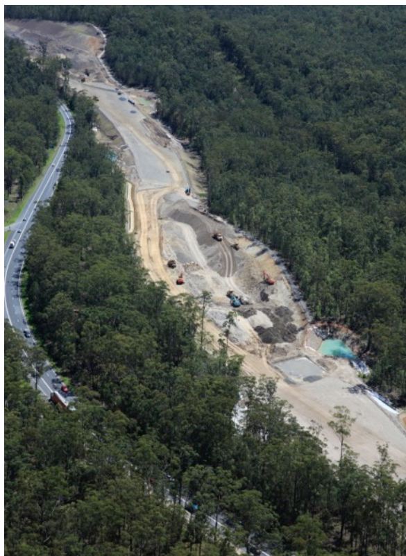
View north along alignment toward deep cutting north of waterway SW11 (St 2)
