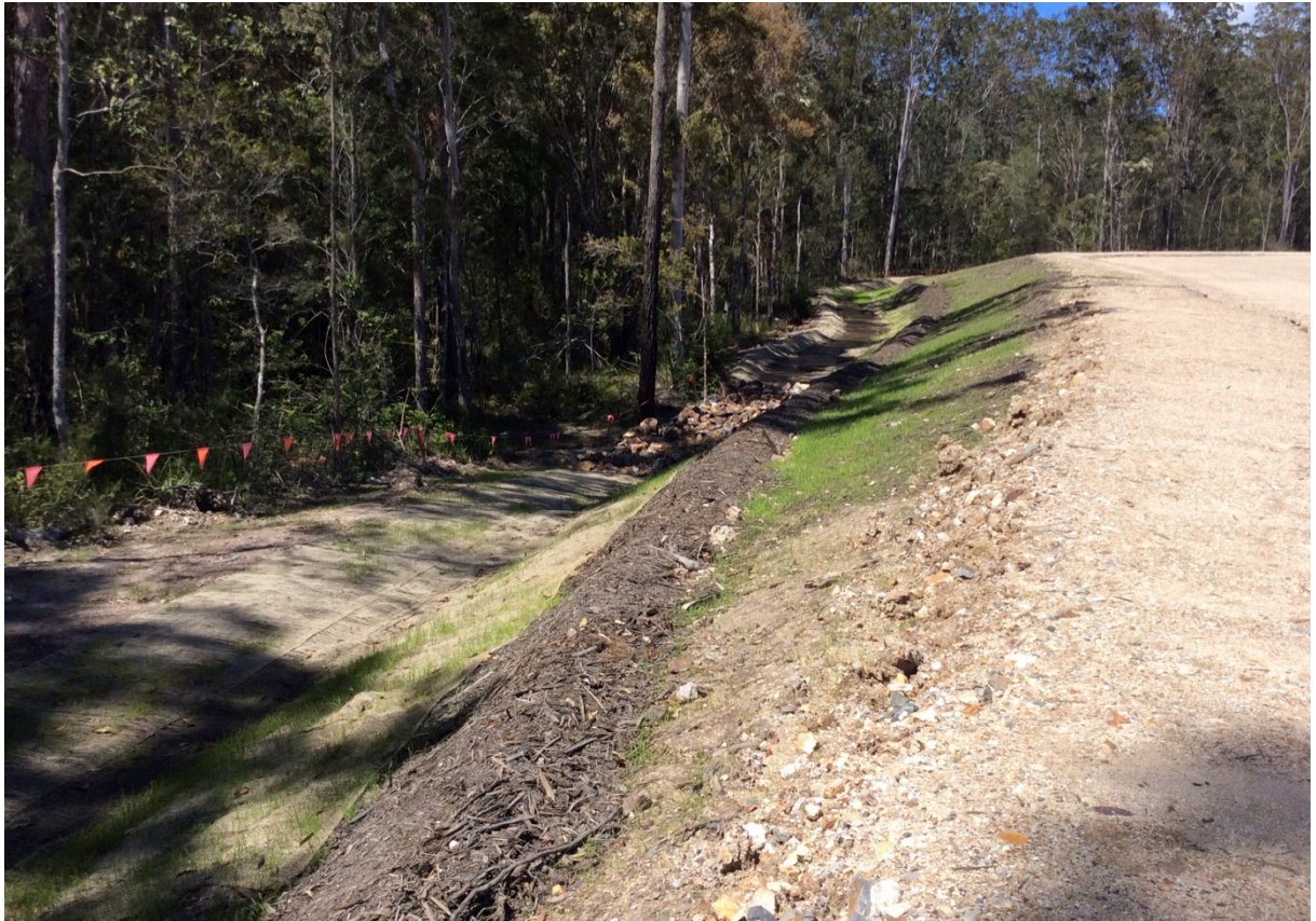
View of batter treatment and temporary ERSED controls on southbound rest area (St 2)
