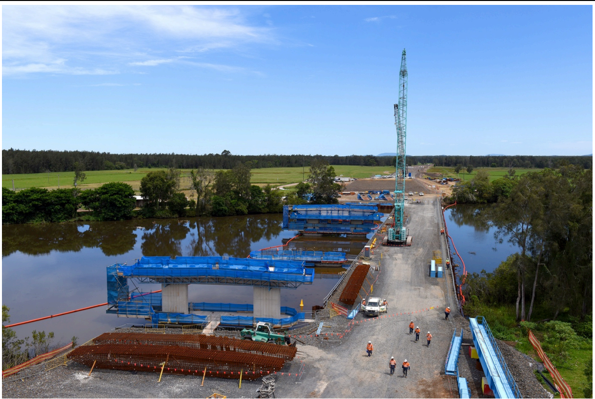
Custom silt curtain around temporary working platform on the south arm of Wilsons River (St 3)
