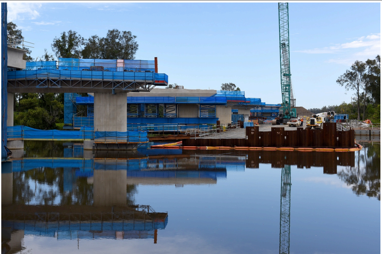
Custom silt curtain around temporary working platform on the south arm of Wilsons River (St 3)
