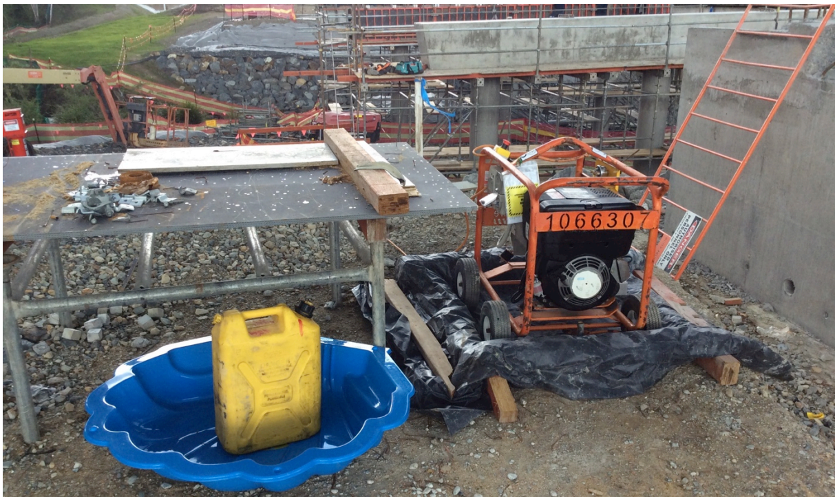
Temporary bunding of pumps and chemicals at Pipers Creek (St 3)
