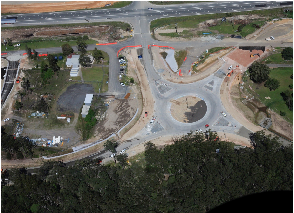
View of northeast roundabout where access is provided to Cassegrain Winery (St 1)
