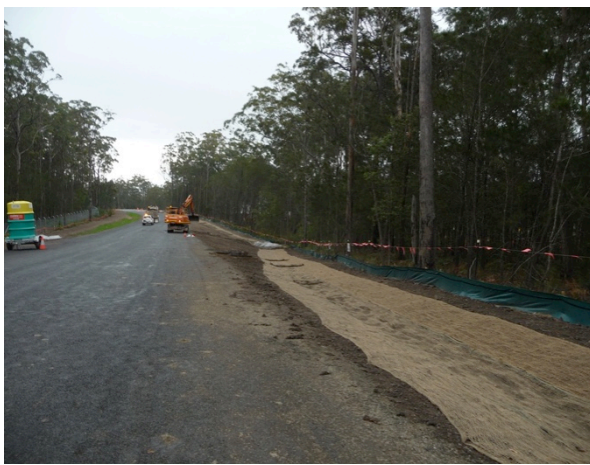
Preparation of table drain on Service Road 3 with topsoil and jute mesh (St 1)
