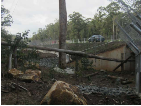
Figure 11 Koala rails and refuge poles at dedicated fauna underpass, Oxley Highway (Source: SHJV)
