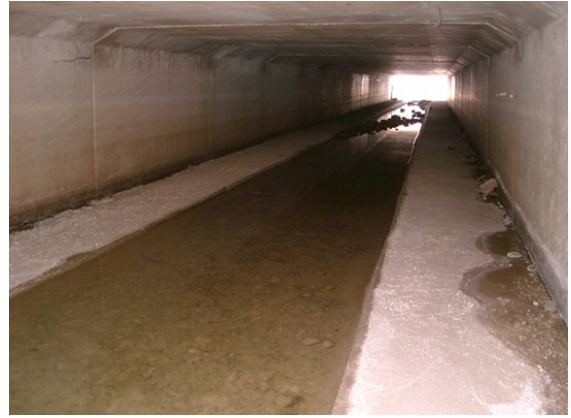
Figure 6 Combined fauna underpass culvert with shelf for dry passage, Pacific Highway upgrade (Source: RTA 2010)
