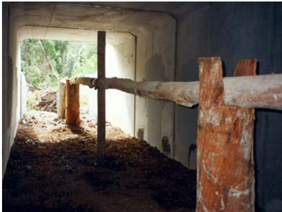
Figure 13 Koala rails in underpass at Sapphire to Woolgoolga Pacific Highway upgrade (Source: RTA 2010)
