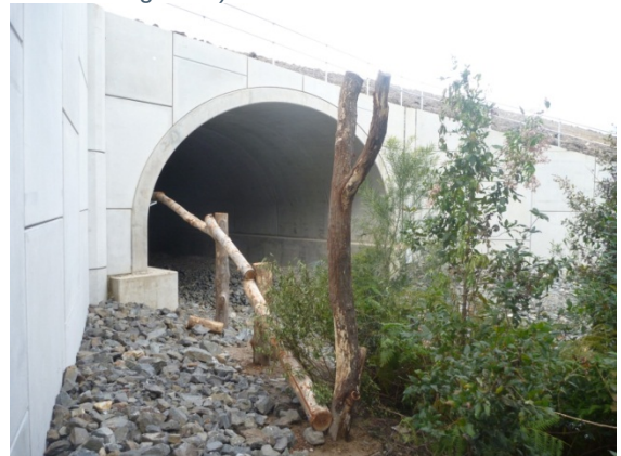
Figure 14 Koala rails in Boat Harbour Creek combined culvert, Kempsey Bypass (Source: Lewis Ecological Consulting 2012)
