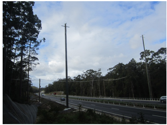
Figure 2: Example of glider poles at Oxley Highway (Source: Laura Worthington, Hyder Consulting)
