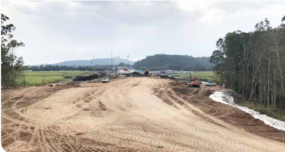
Work progressing on the southern approach to the new bridge over the Richmond River
