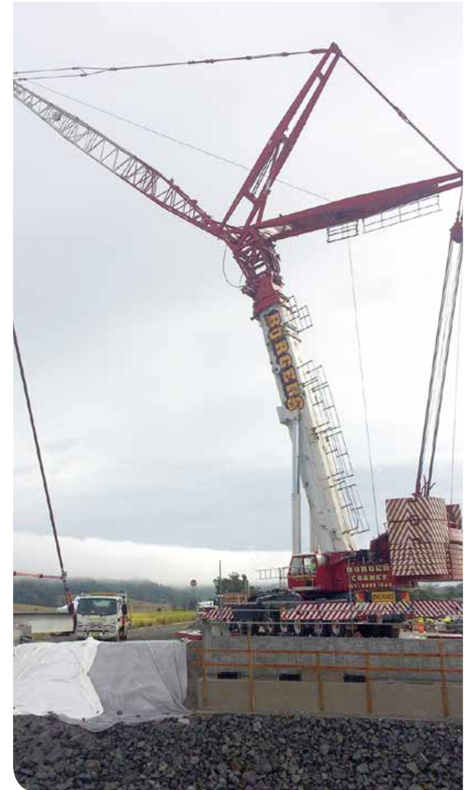
Installing girders for the bridge north of Old Bagotville Road at Bagotville
