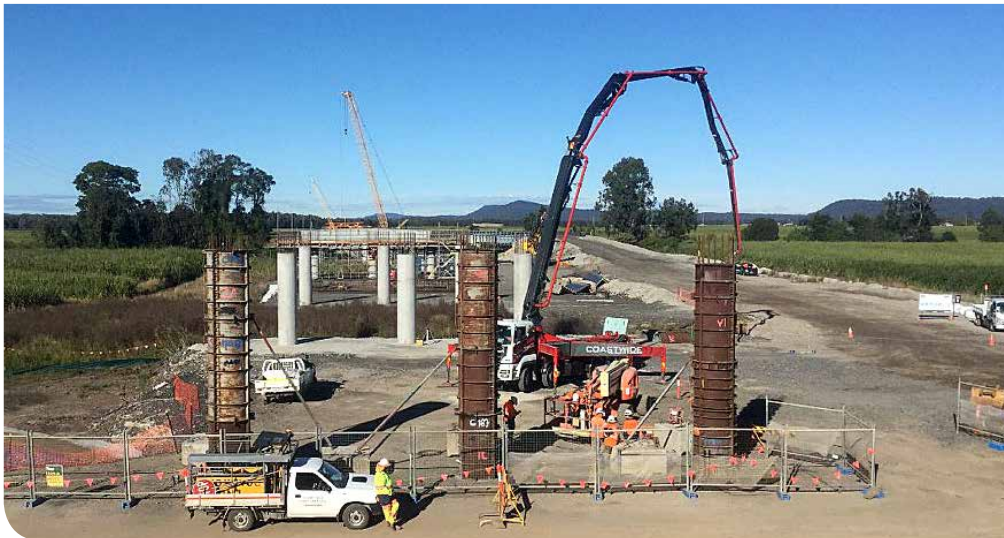
Pier forms ready for concrete pour for the new bridge over Shark Creek at Shark Creek
