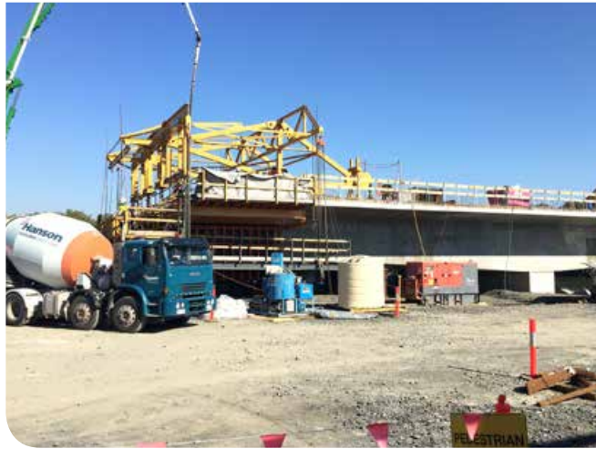
Building deck segments on the balanced cantilever bridge over Emigrants Creek at Pimlico
