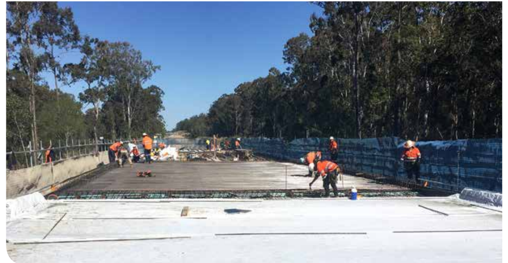
Preparing for a deck pour at bridge near Darky Road at Tabbimoble
