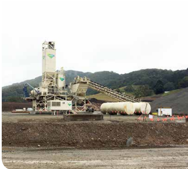
Temporary concrete batch plant construction completed for work between Broadwater and Pimlico
