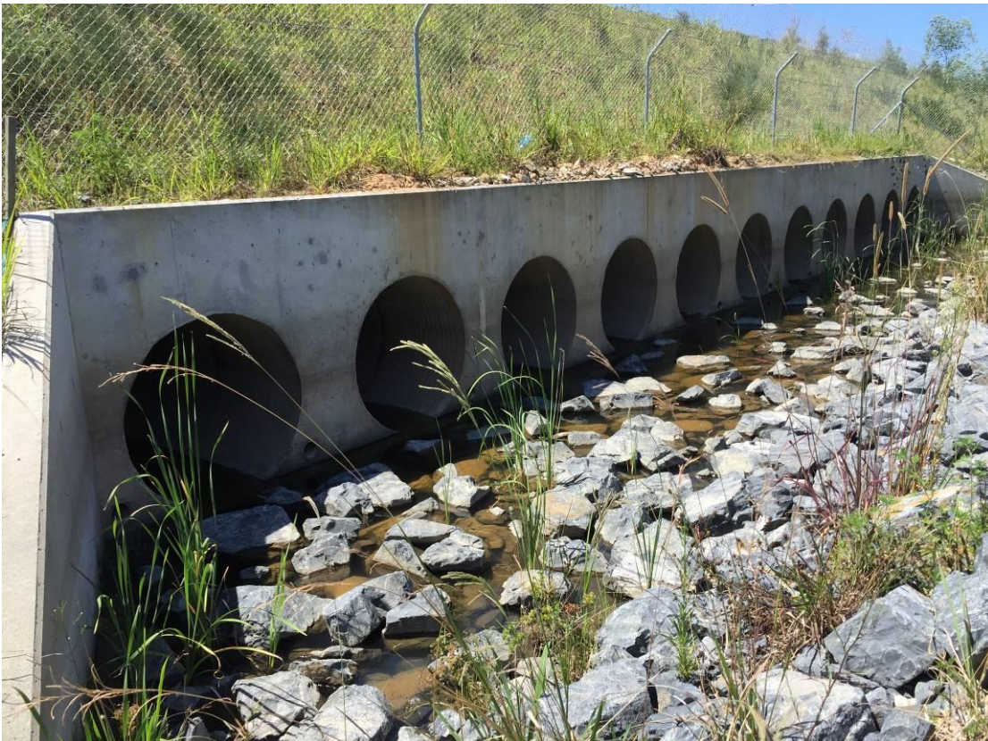
Plate 9: Emerald Beach underpass (ch.17500) viewed from the east (upper) and west (lower).
