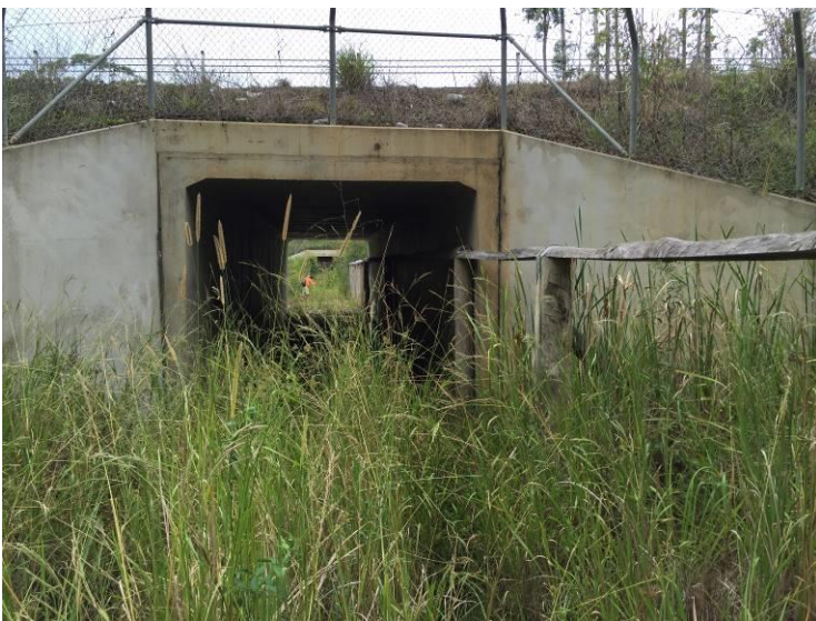
Plate 11: Arrawarra underpass north (ch.29930) viewed from the east (upper), across the vegetated median (middle) and from west (lower).
