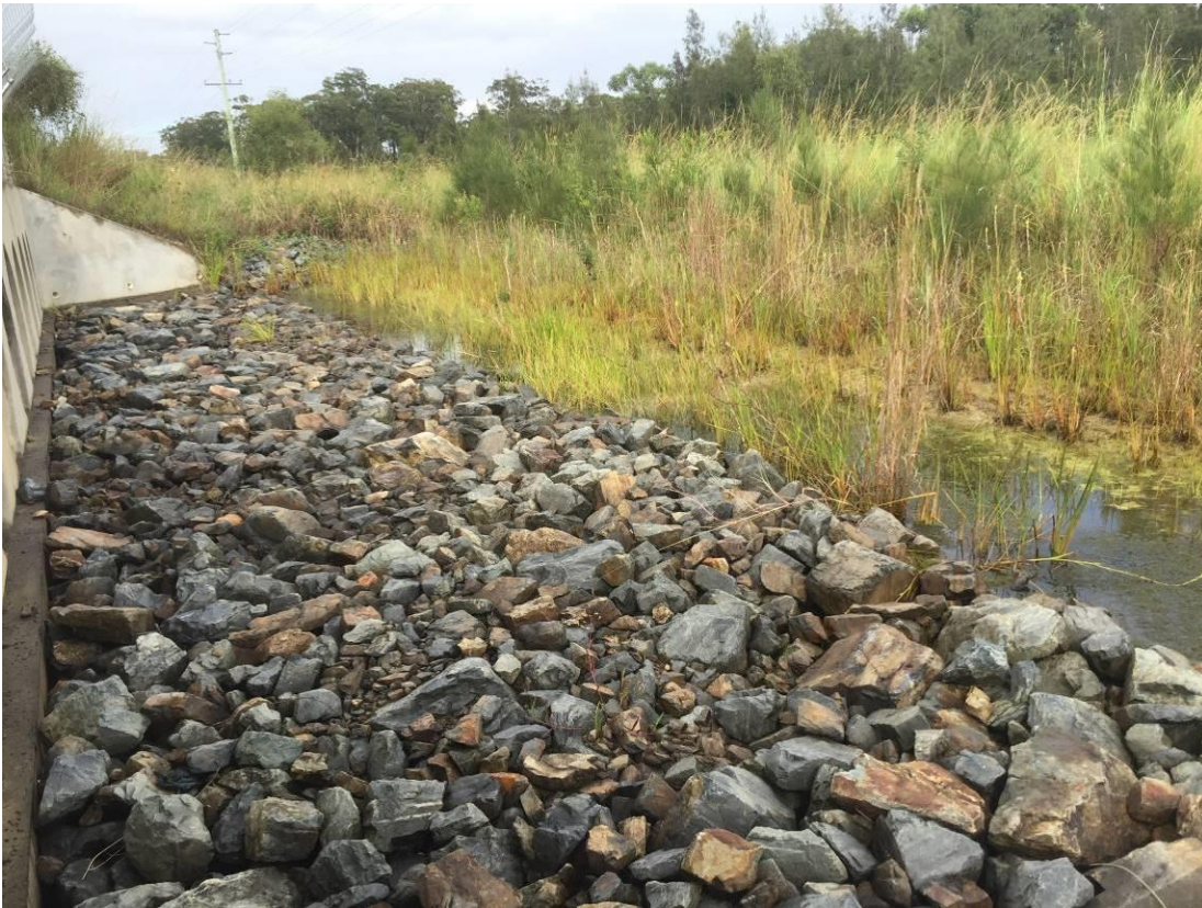
Plate 3: Habitat adjoining Emerald beach underpass (ch.17500) on the east (upper) and west (lower) side of the alignment.
