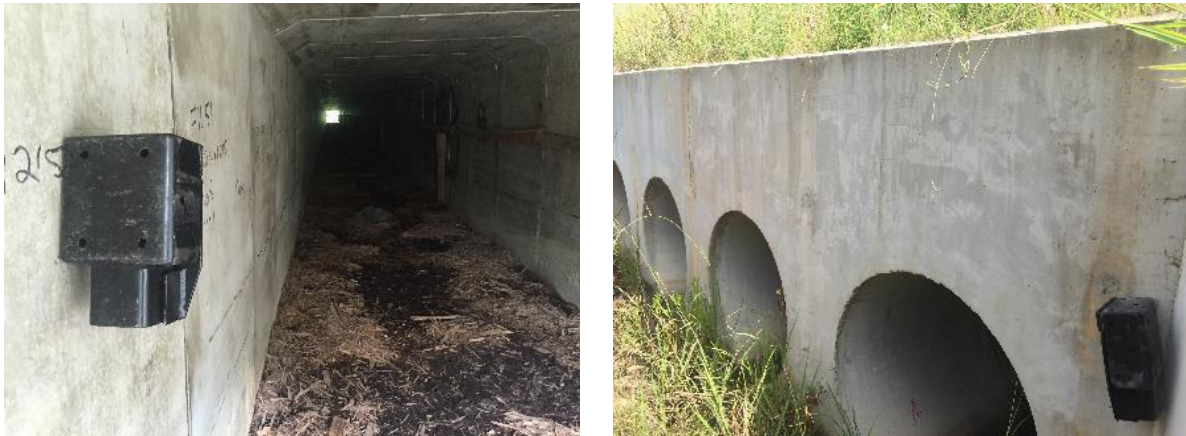
Plate 12: Single cell underpasses were monitored at each end with a Reconyx HC500 camera housed in a security case and mounted to the side wall opposite the wooden rail (e.g. Moonee underpass, Left). For the pipe series at Emerald Beach, a camera was mounted on the wing wall at each end of the pipe series and directed across the entrance area of the east side (Right).
