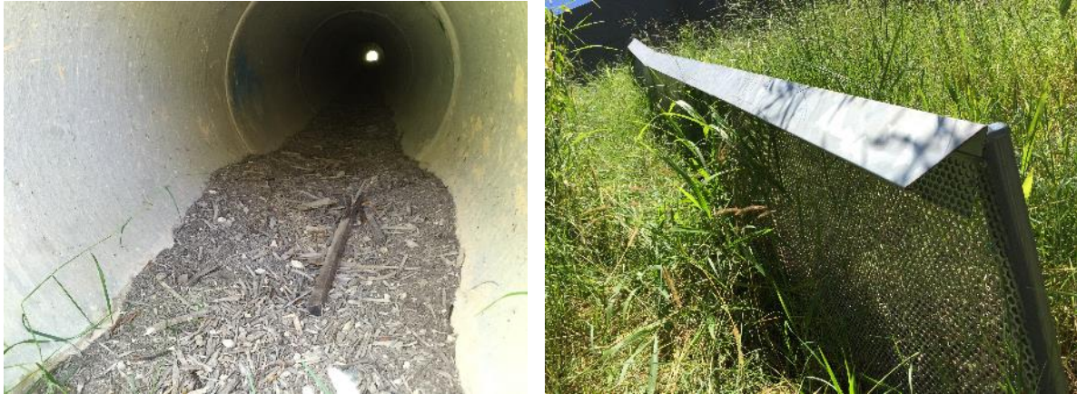
Plate 5: Pipe inverts/floors were covered in 50-100mm thick mulch (L). Frog exclusion fencing extended up to 20m beyond pipe wing-walls (R). (Picture taken 19 November 2015)
