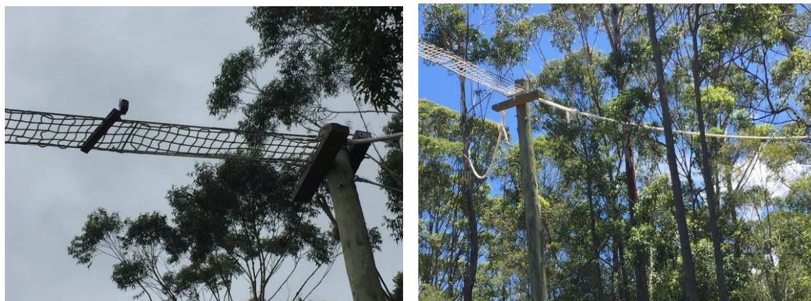
Plate 15: A Reconyx camera mounted to a wooden ‘sandwich board’ was positioned approximately 2m from each end of the rope bridge to capture moving fauna (L). Slung rope (25mm diam.) was used to link the bulkhead to surrounding trees (R).
