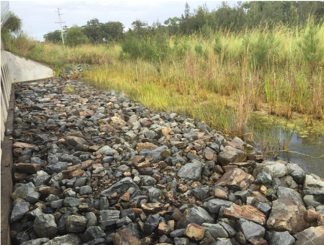
Plate 3: Habitat adjoining Emerald beach underpass (ch.17500) on the east (top) and west (bottom) side of the alignment.
