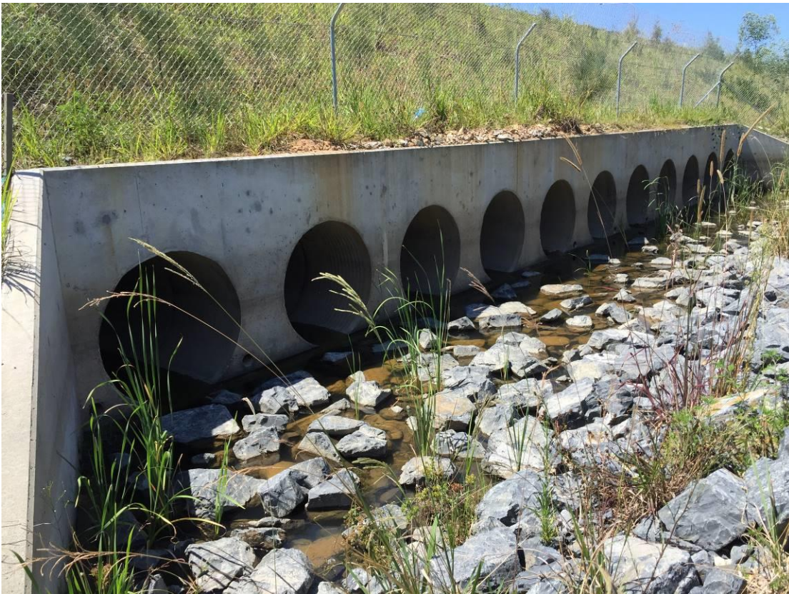
Plate 9: Emerald Beach underpass (ch.17500) viewed from the east (top) and west (bottom).
