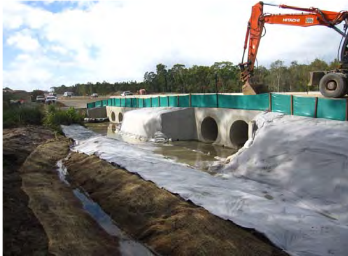
Photo - Triple and double cell culverts south of Gate 13C with associated erosion and sediment controls.
