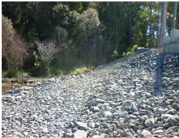
Photo – Installed scour protection and fauna passage at Skinners Creek with smaller rock
