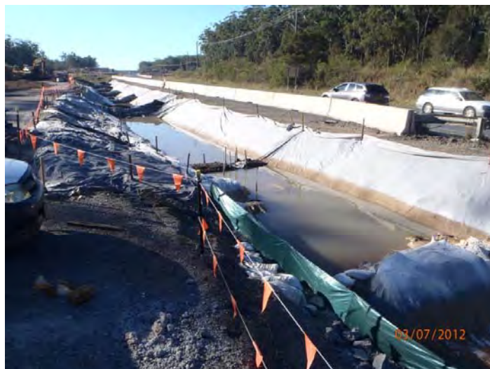
Photo – Proactive management of site water north of Arrawarra Creek near Nashs Road, using combined rock/ mulch controls, lining and gypsum to reduce water quality impacts.
