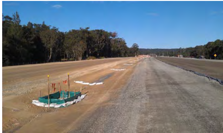
Photo – Inlet pit and median erosion and sediment controls to minimise sediment impacts between Smiths Road and Killara Avenue
