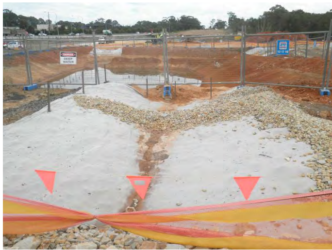
Photo - Gypsum used at the inlets of all basin to mix with stormwater to assist in quick flocculation and releases
