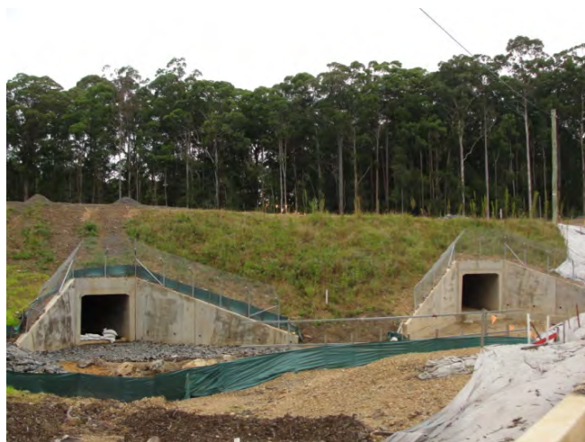
Photo - Higher level fauna underpass culvert on the right, lower level drainage culvert on the left.
