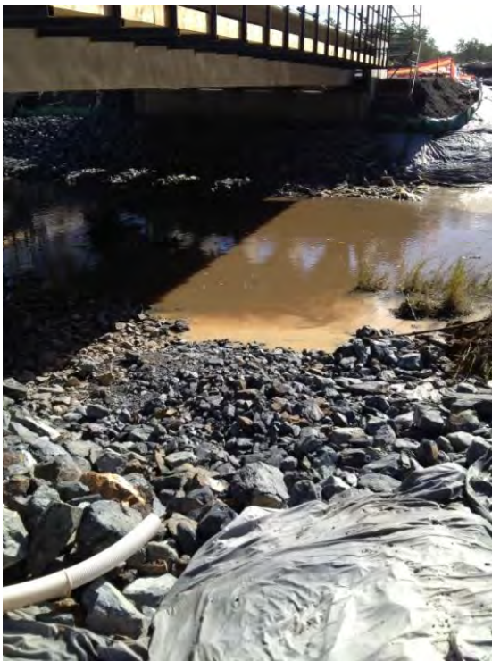
Photo 2: Colloidal material bleeding through bridging at Arrawarra Creek.
