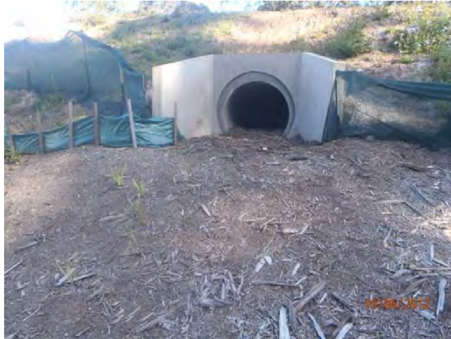
Photo – Giant Barred Frog culvert located north of Greys Road bridge site (to be fitted with motion sensors and video equipment)
