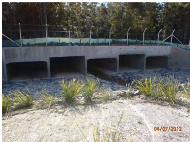
Photo – Fish passage at culvert 30.05/06 in Wedding Bells area also showing planted Lomandra's in the waterway area
