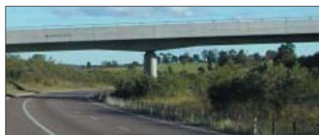
Illustrations 88-90: Examples of haunching and pier design well integrated (88-89) and poorly integrated (90) (source: RTA ' Bridge Aesthetics ', p 27)
