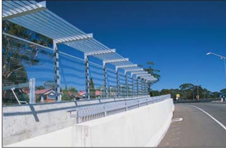
Illustration 99: An example of an integrated barrier and safety/ throw screen design near Shell Corner, on the Great Western Highway.
