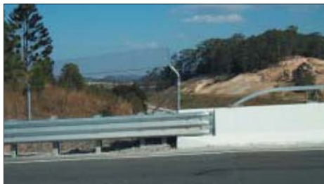
Illustration 95: This design detail has successfully integrated a safety barrier and bridge parapet (source: RTA 'Bridge Aesthetics', p 43)
