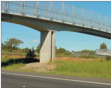
Illustration 91: The thickness of the pier on this bridge has been broken up by the use of a shadow recess, reducing the perceived thickness of the pier (source: RTA 'Bridge Aesthetics', p 8)
