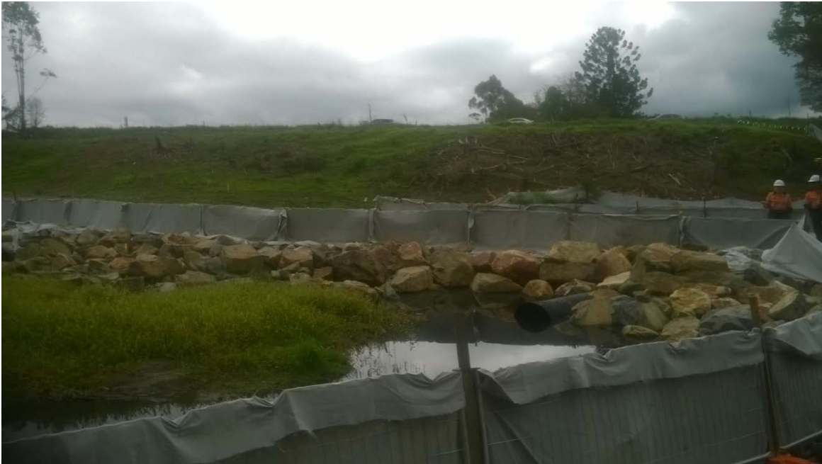
Photo 9: Frog fencing (southern zone)
