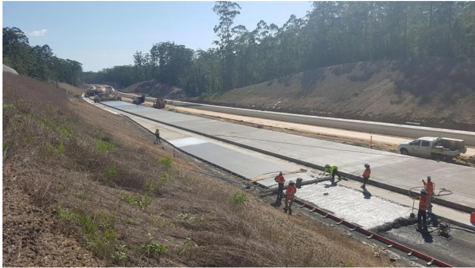
Photo 1: Paving operations have commenced with both base and sub-base concrete pavement installed
