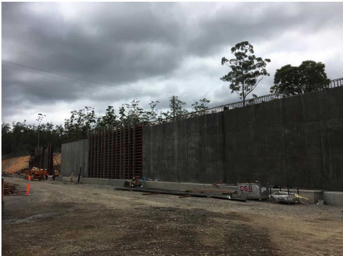
Photo 2: Construction on the railway underpass has commenced, the cut has been excavated and the concrete walls are under construction.
