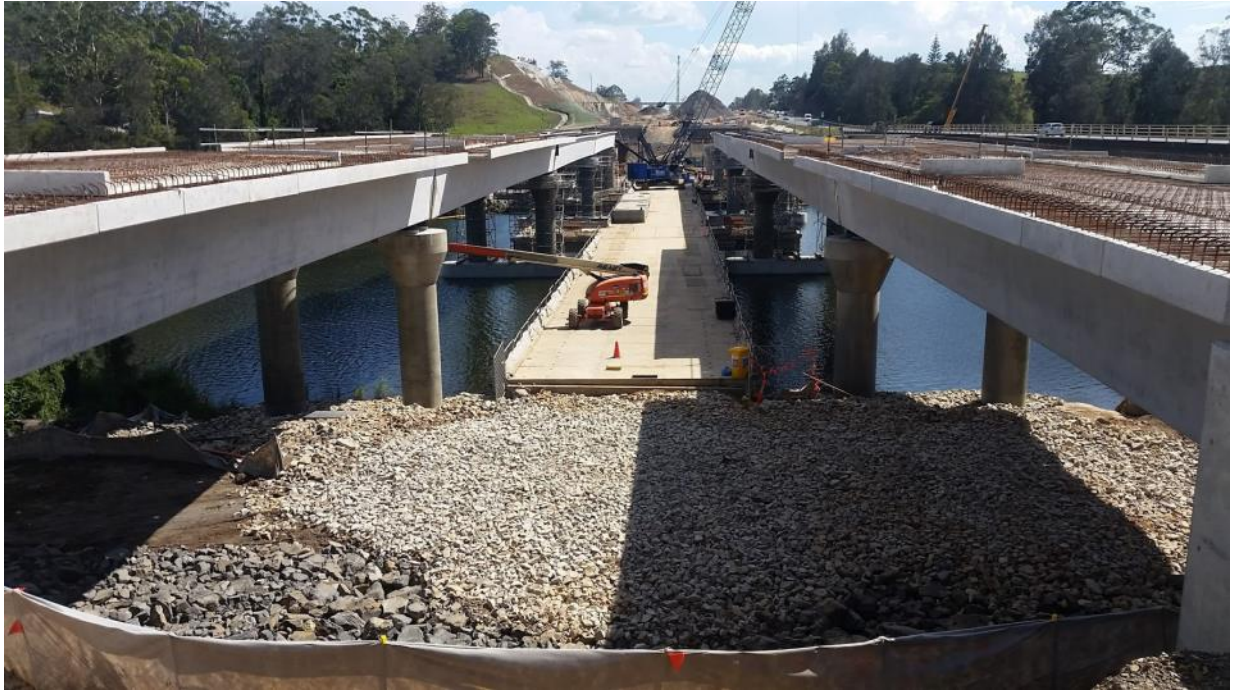
Photo 3: A temporary bridge was used to construct the twin bridges over Lower Warrell Creek; this helped to reduce the impact of construction activities on the creek (including reducing the requirement for rock platform construction).
