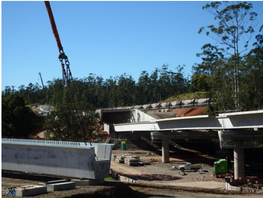
Photo 1: Girder installation on Upper Warrell Creek. All girder placements are complete for the Project.
