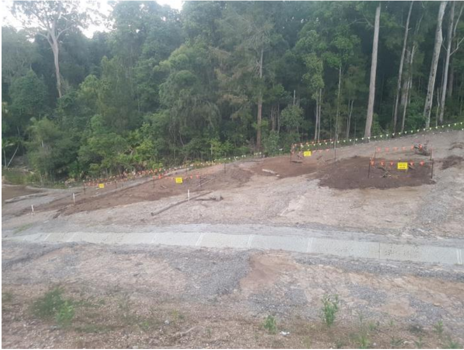
Photo 2: Construction of frog breeding ponds in accordance with the Green-Thighed Frog Management Plan
