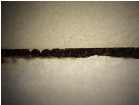
Plate 1.1 Culvert 599205 - Deadman's Gully. Approx. 1000 M. australis in segment gaps.
