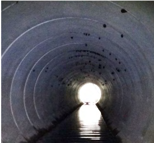
Plate 1.1 Structure ID 37 (599205) - Deadman's Gully pipe culvert: approximately 400 Eastern Bentwing Bats in segment gaps.
