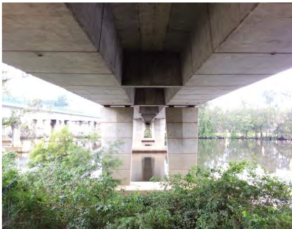
Plate 1.3 Lower Warrell Creek Bridge Structure ID 21 (1871): northern abutment recorded guano and staining beneath.
