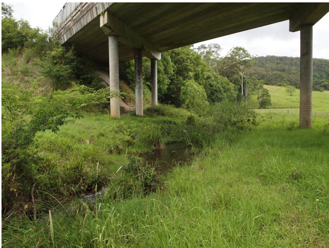
Plate 9: Williamson's Creek looking east under the existing Pacific Highway bridge; there was no Maundia in the section of the creek beneath the bridge and to either side for 20-30 metres.
