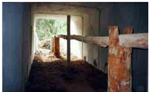
Plate 2 Example combined fauna / drainage structure
