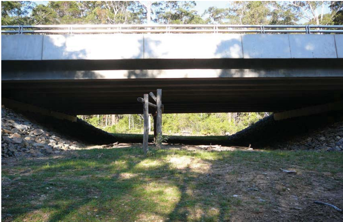
Fig 5: Fauna Underpass bridge at Pacific Highway Bonville Upgrade . . Results from AMBS monitoring have shown koalas using this underpass
