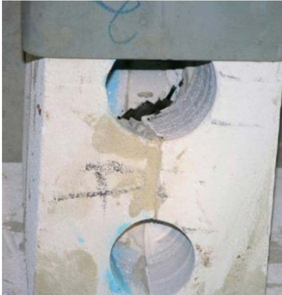
Plate 3.9 Lightweight concrete blocks with drill holes, microbat visible in chamber (Source: N Williams)
