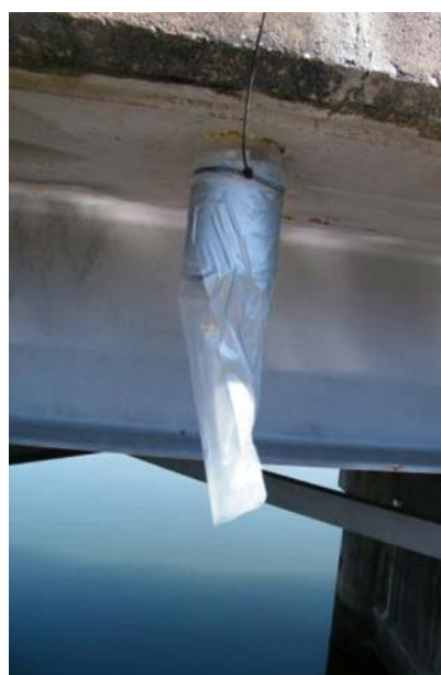
Plate 3.6 Exclusion – Plastic over scuppers (Source: D Andrighetto)
