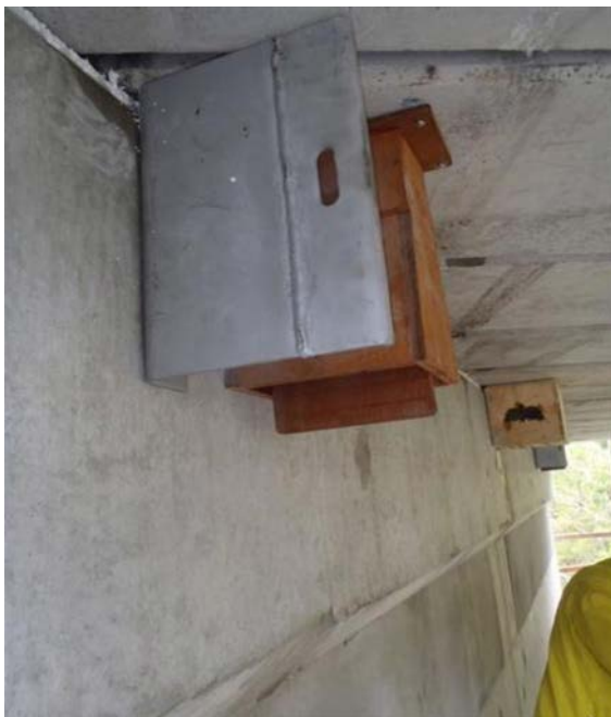
Plate 3.7 Bat boxes with bash plate beneath Myott Bridge (Source: A Lloyd)
