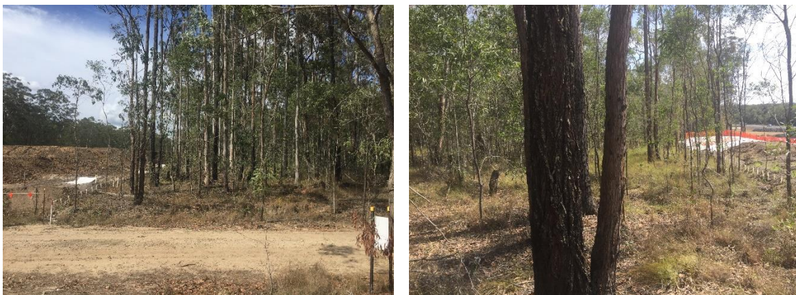
Plate 1: At the time of the surveys, mainline clearing had only occurred adjacent one transect, TabN-cw, in the vicinity of Glencoe Road at the edge of Tabbimoble State Forest. Both plates show the 40m-wide forest strip remaining between the transect and mainline clearing.
