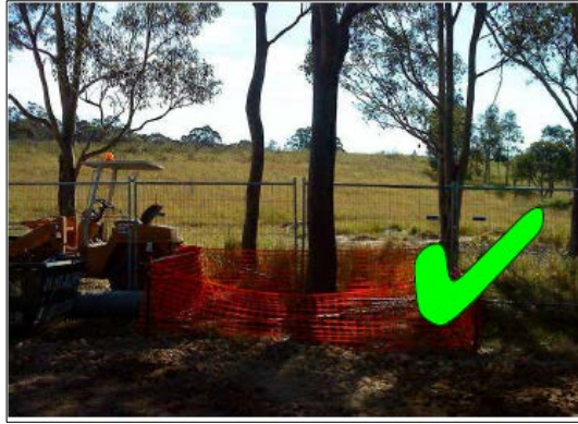
Figure 4: Tree protected via fencing with no materials stored within the drip line.
