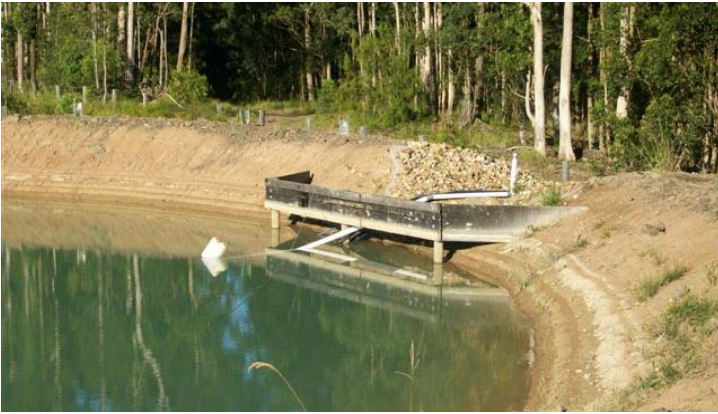
Figure 5. A siphon and float system used for discharging a basin without use of pumps. Floats may be useful for preventing inlets from falling into sediment zones.
