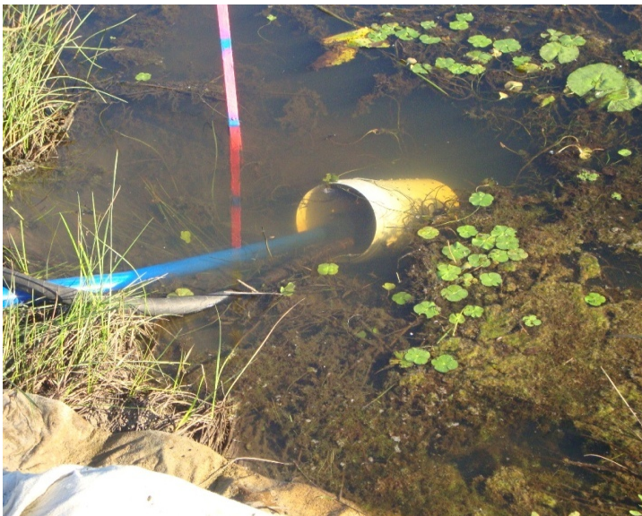
Figure 2. Consideration should always be given to measures to prevent pumped inlets from falling into sediment zones at the bottom of basins. In this example an anchored bucket was seen to be effective.
