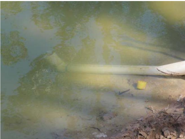
Figure 6. An inlet designed with up-turned pipe to ensure settled sediment is not sucked up during discharge. Note that sediment storage zone needs regular maintenance to ensure levels do not reach the inlet level.
