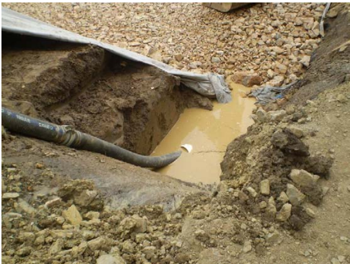
Figure 4. A sump adjacent to a working area may require higher levels of maintenance in order to remain effective. Dewatering to a larger sediment basin will be a more viable treatment measure when compared to flocculating the sump itself. Consideration to minimising exposed fines around the immediate catchment (e.g. bottom left corner of the figure) will also reduce sediment entering the sump if deemed practical for construction purposes.
