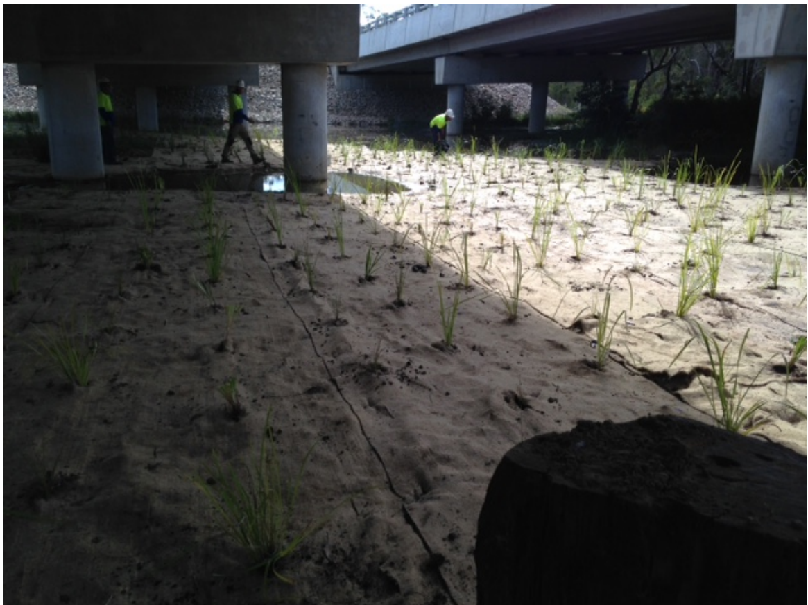
Photo: Wells crossing -jute matting and landscape planting over temporary access platform area following removal in May 2017.
