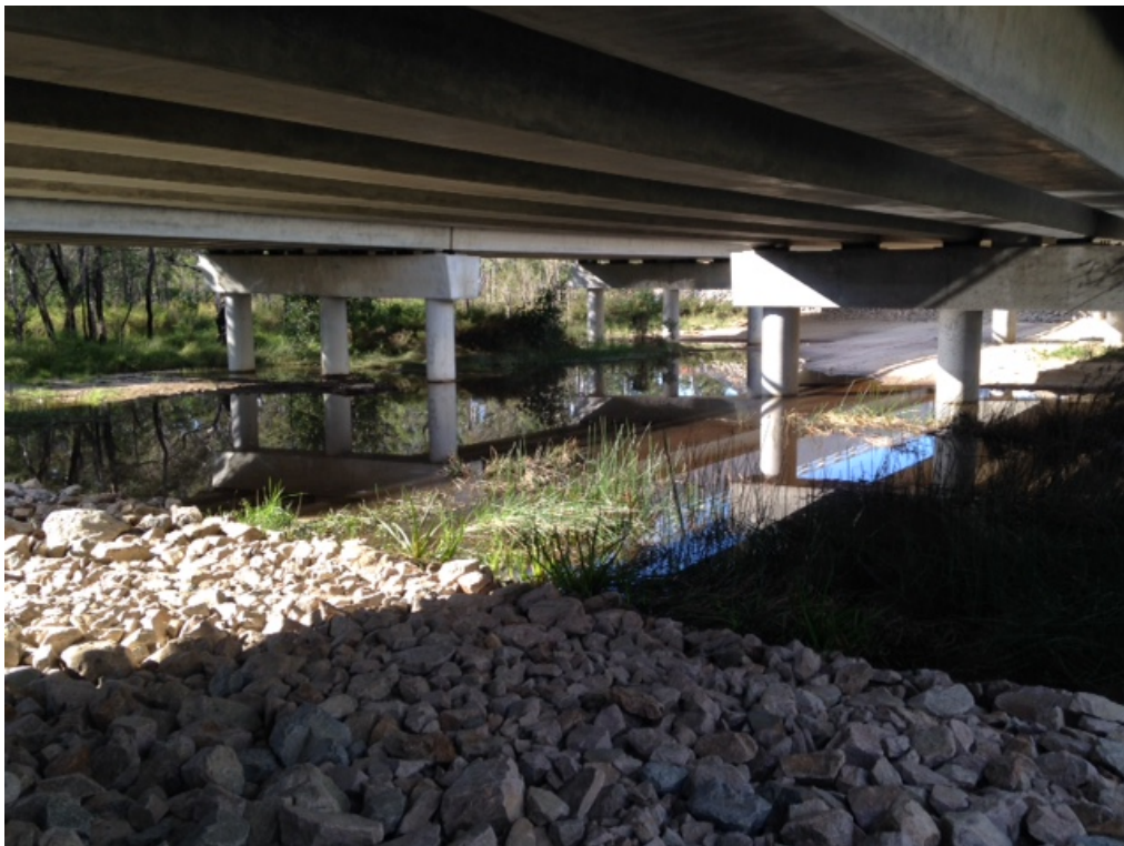
Photo: Wells Crossing June 2017 following removal of temporary access platform between the two bridges in May 2017
