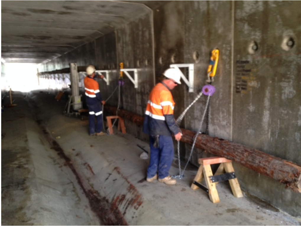
Photo: Stage 1 of innovative process to install large diameter fauna rails into culverts – use of quick hitch (yellow) with block and chains (connected to retained culvert lifting lugs – retained for microbat habitat creation) for initial lift of heavy logs within culvert
