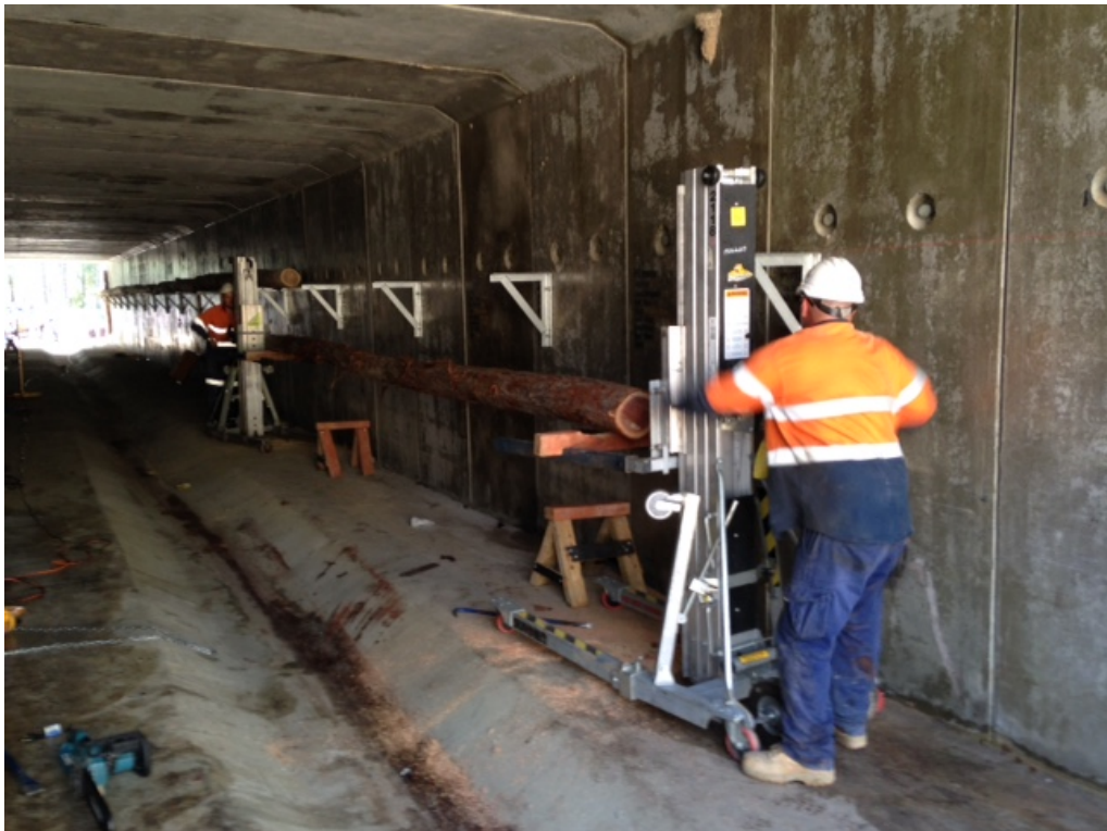
Photo: Stage 2 – utilisation of two garage door lifting rigs to lift to required height and secure to installed metal brackets
