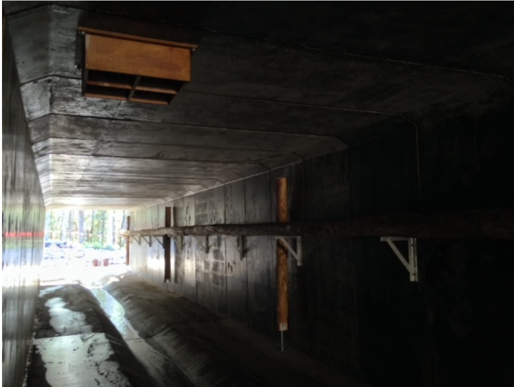
Photo: finished product showing (i) horizontal fauna rail for arboreal fauna (ii) regular vertical poles to allow transfer to/from rail at multiple points and (iii) hardwood microbat box (installed concurrently with fauna rail installation)
