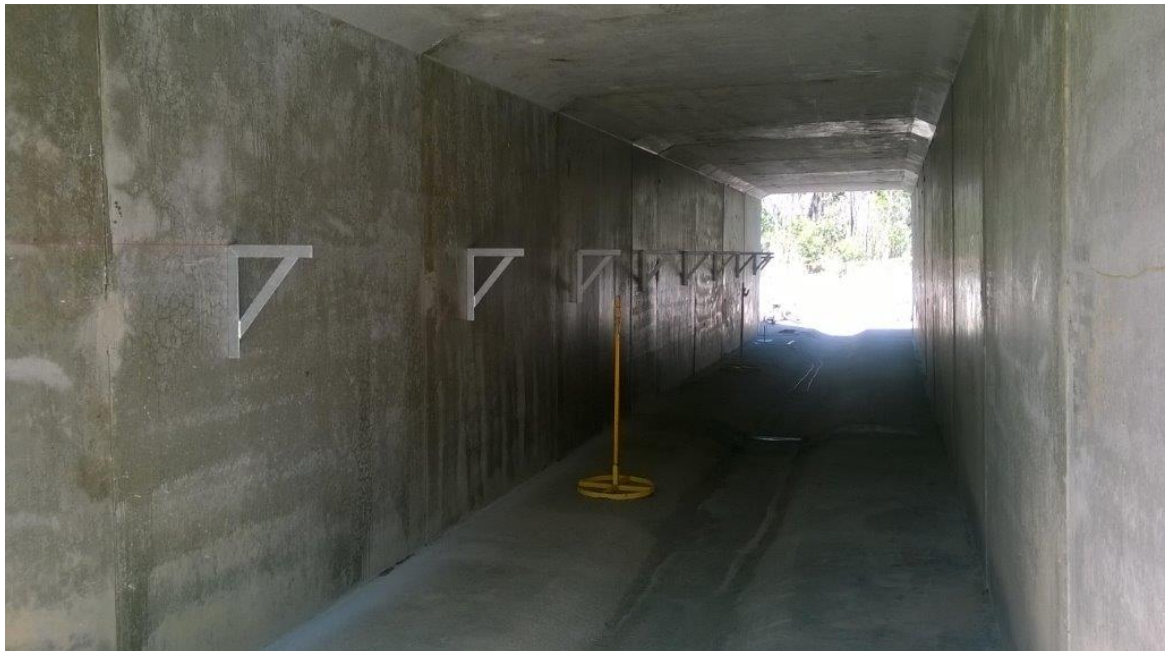
Photo: metal brackets installed in combined drainage fauna underpass in preparation for installation of log rail for passage of arboreal fauna
