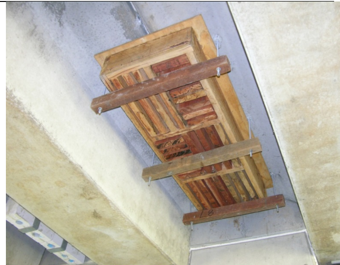
Plate 3.12 Lattice style bat box under bridge (Source: N. Williams)
