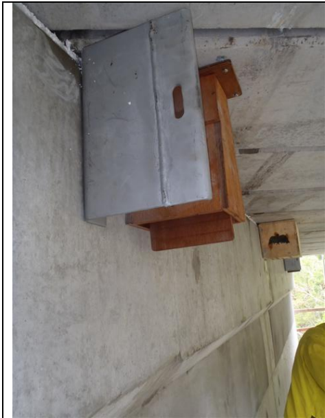
Plate 3.7 Bat boxes with bash plate beneath Myott Bridge (Source: A. Lloyd)
