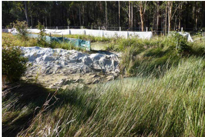
Evidence of recent high water flows, damage to protective matting
