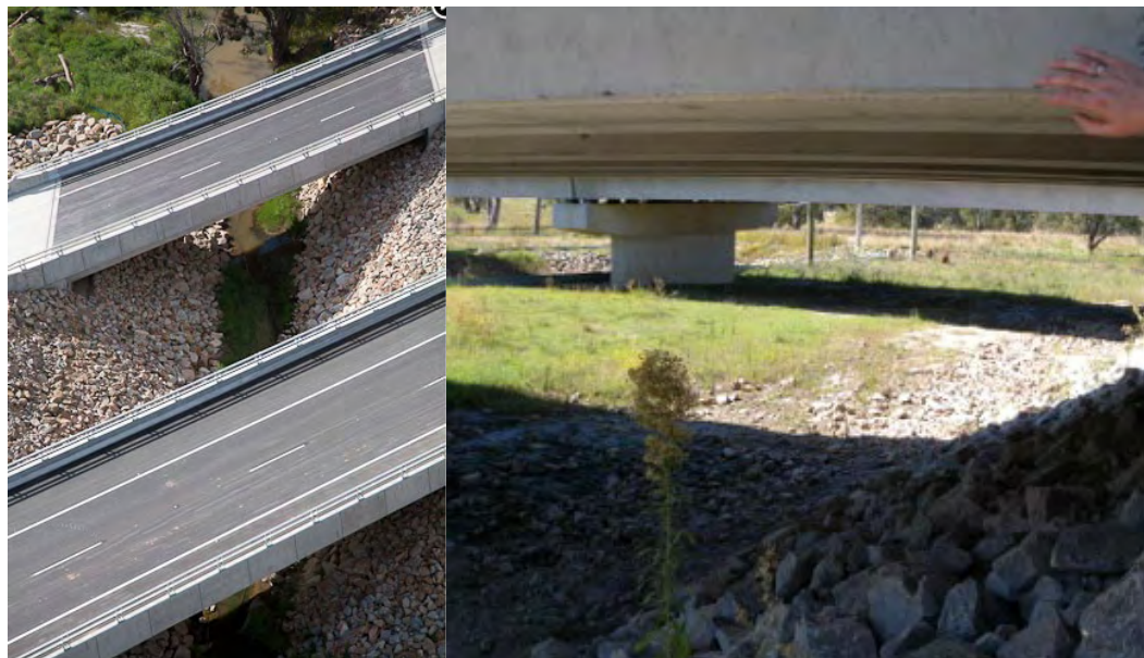
Plate 6.5: Retention of existing creek invert and floodplain at the Hume highway Woomargama Bypass (Source: HHWA)
