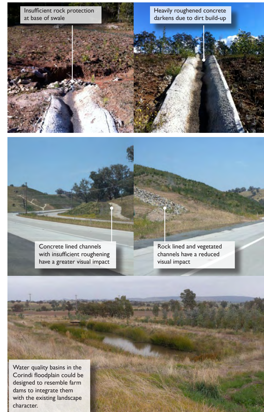
Plate 6.9: Drainage elements at Pacific Highway Glenugie upgrade (top) (Source: SMM and Roads and Hume Highway Woomargama Bypass (middle and below) (Source: SMM and Roads and Maritime)
