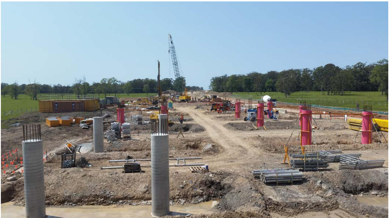
Looking south at piling work under way for the Corindi floodplain twin bridges (November 2015)
