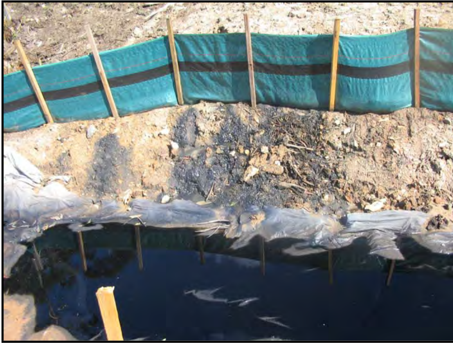
Plate 5: Tannins in a drainage line generated from very thickly applied mulch on the batter above. Note that the sedimentation fence is not effective in treating the tannins.
