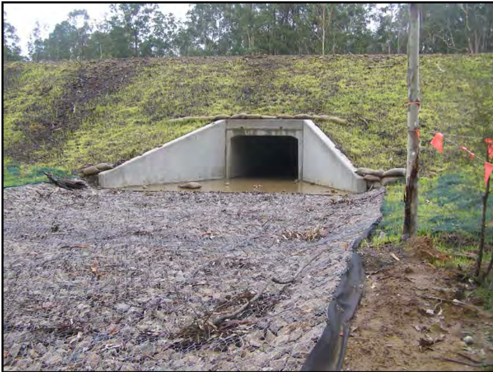
Plate 9: A mulch/topsoil mix used to provide temporary batter stabilisation and to assist cover crop establishment.
