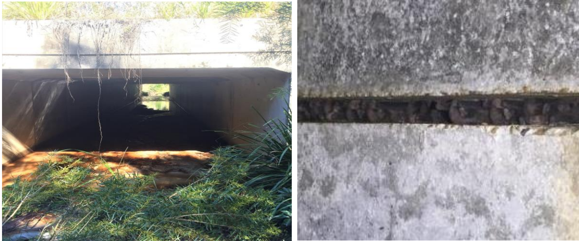
Plate 3: The middle cell of the non-excluded triple cell box culvert #66 (L). The culvert featured approximately 505 little bent-wing and five Eastern bent-wing bats during autumn and winter inspections (R).
