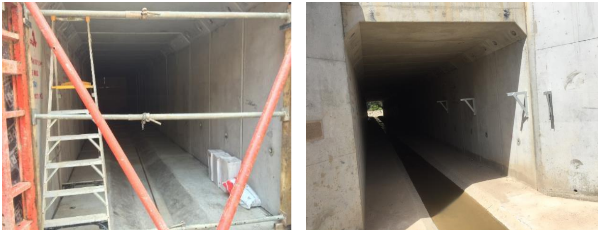
Plate 2: Western view of culvert #49 whilst under construction during autumn inspection (17/5/2017) (L) and 5 months later the complete culvert (26/10/17) (R)
