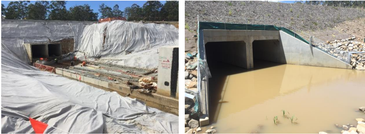
Plate 1: Western view of culvert #46 (Boney's Creek) during construction of the new culvert (17/5/2016) (L) and the same view of the completed culvert during the spring survey (26/10/17) (R).
