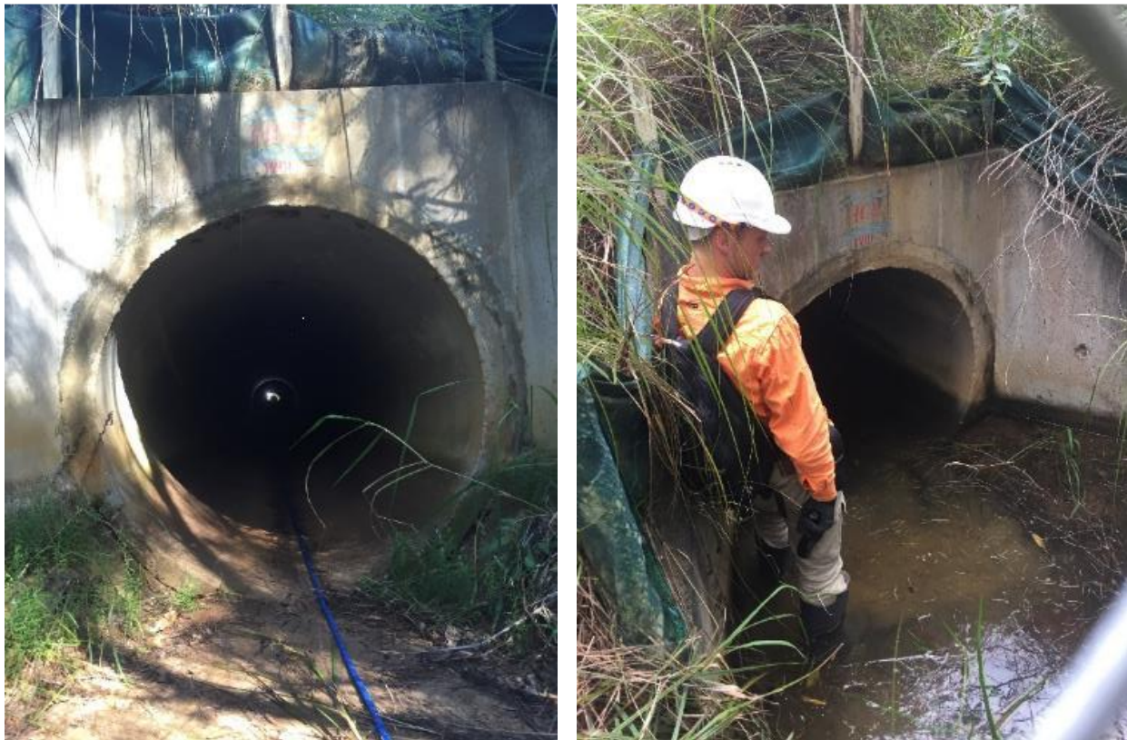
Plate 4: Non-excluded RC pipe #67 featured a single eastern horseshoe bat during summer and autumn (left). Approximately 400mm of water flowed through the pipe during winter (right).
