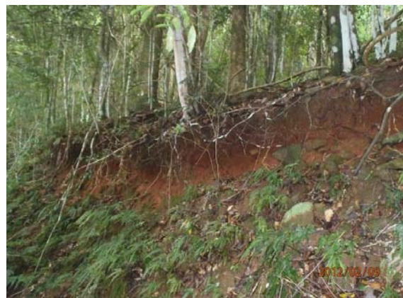
Photo 4. Overhang at site 9.
