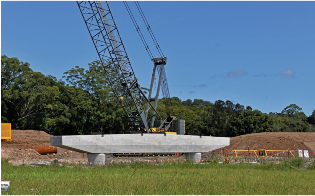
The first headstock installed on the southern side of the Richmond River
