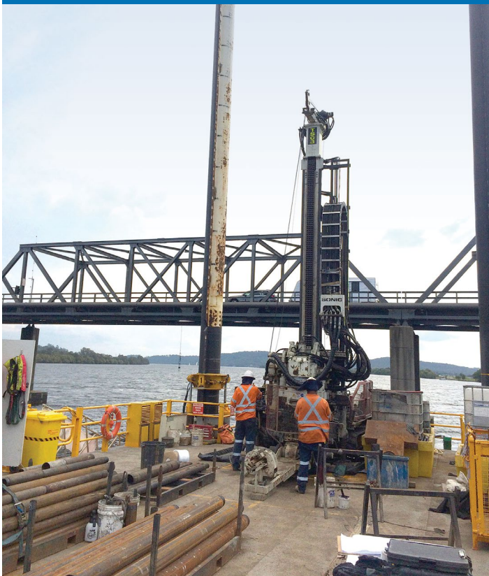
Example of drilling rig being operated for geotechnical investigations at the new bridge over the Clarence River at Harwood
