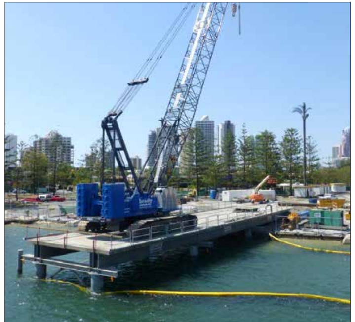
An example of the temporary jetty to be used at River Street
