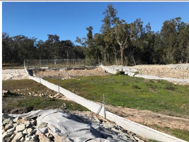
Plate 4 Eastern end of run viewed from northern edge. Note haul road in the far left (eastern edge) and creek is to the west (right). (Source: Seymour Whyte, August 2017).
