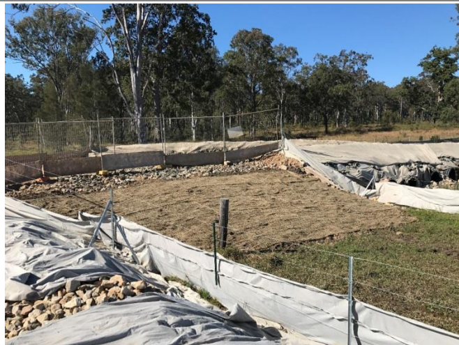
Plate 15 Western batter of haul road at the eastern end of the run. (Source: Seymour Whyte, August 2017).
