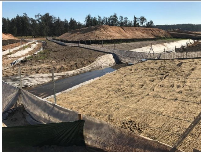
Plate 10 Emu run from the eastern haul road batter. (Source: Seymour Whyte, August 2017).
