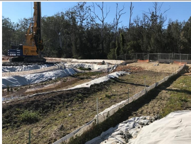
Plate 13 Western batter of haul road at the eastern end of the run. (Source: Seymour Whyte, August 2017).
