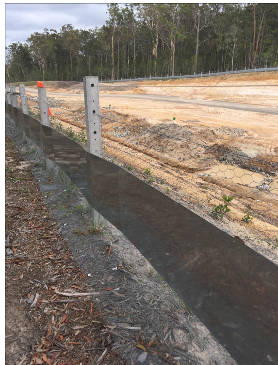
Plate 10. Permanent emu exclusion fence erected adjacent to crossing zone T9 on both sides of the highway
