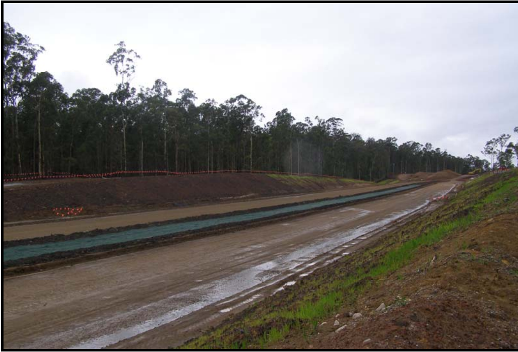
Plate 8: Site showing recent application of a mulch/topsoil mix on batters (40% mulch to 60% topsoil). Mulch mixes are used to provide temporary stabilisation to prevent the loss of topsoil from batters in heavy rainfall events. Mulch use is also shown as a mounded sedimentation control to prevent sediment entering the median drain.
