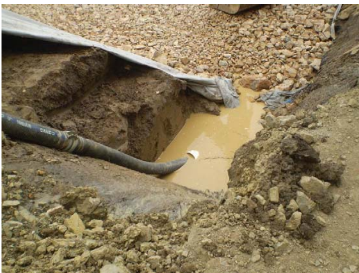
Figure 4. A sump adjacent to a working area may require higher levels of maintenance in order to remain effective. Dewatering to a larger sediment basin will be a more viable treatment measure when compared to flocculating the sump itself. Consideration to minimising exposed fines around the immediate catchment (e.g. bottom left corner of the figure) will also reduce sediment entering the sump if deemed practical for construction purposes.
