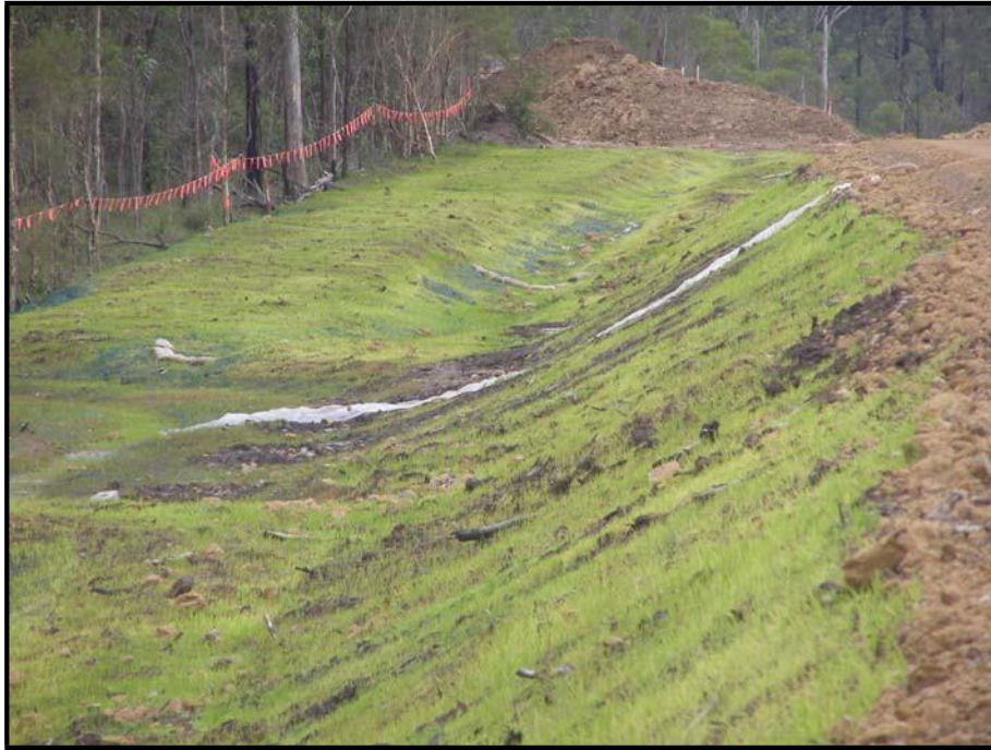
Plate 10: Successful establishment of cover crops on batters where mulch has been used with topsoil to assist temporary stabilisation.
