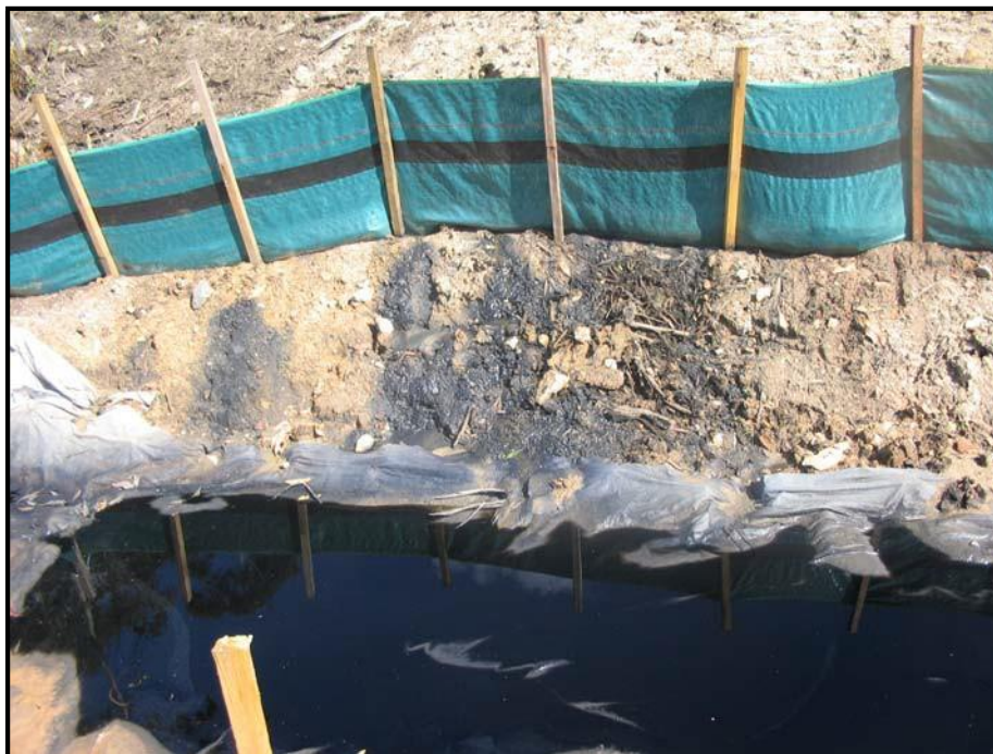
Plate 5: Tannins in a drainage line generated from very thickly applied mulch on the batter above. Note that the sedimentation fence is not effective in treating the tannins.
