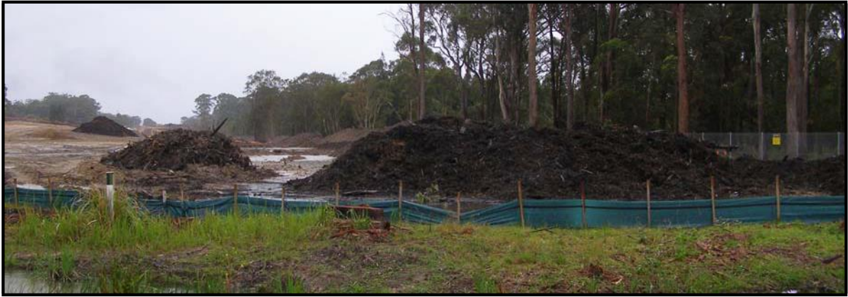
Plate 6: Mulched vegetation stockpiled in a low-lying area subject to inundation. This is not an appropriate stockpile location and may increase the generation of tannins from stockpiled mulch.
