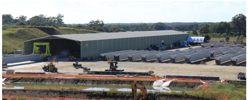
Pre-cast facility and storage area at the Warrell Creek to Nambucca Heads Pacific Highway upgrade
