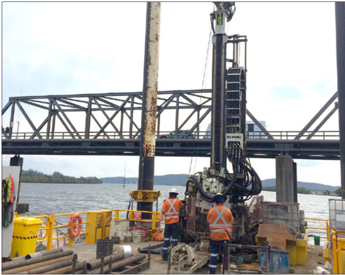
Geotechnical investigations in progress for the new bridge over the Clarence River at Harwood
