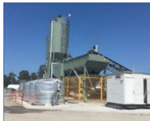
Temporary batch plant at Avenue Road, Pillar Valley for the Woolgoolga to Ballina Pacific Highway upgrade
