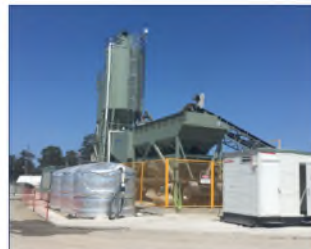
Temporary batch plant at Avenue Road, Pillar Valley for the Woolgoolga to Ballina Pacific Highway upgrade
