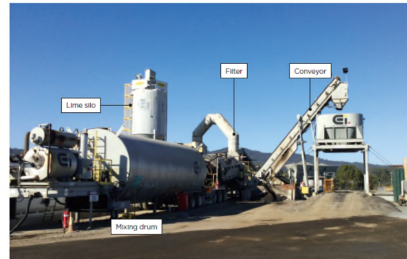
Temporary asphalt batch plant for the Warrell Creek to Nambucca Heads section of the Pacific Highway upgrade
