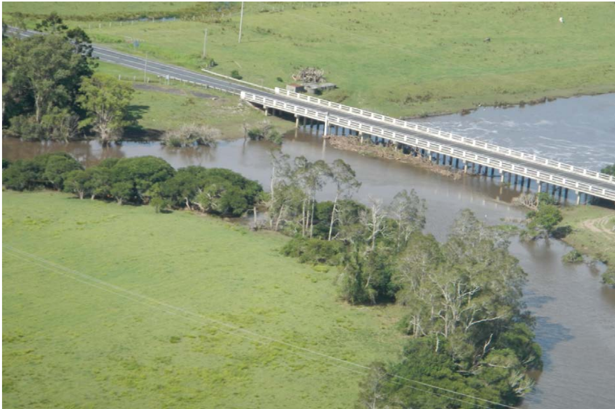
Plate C -9 Tuckombil Canal (1 February 2013, 3.20pm), showing moderate to major evidence of debris blockage around bridge piers.
