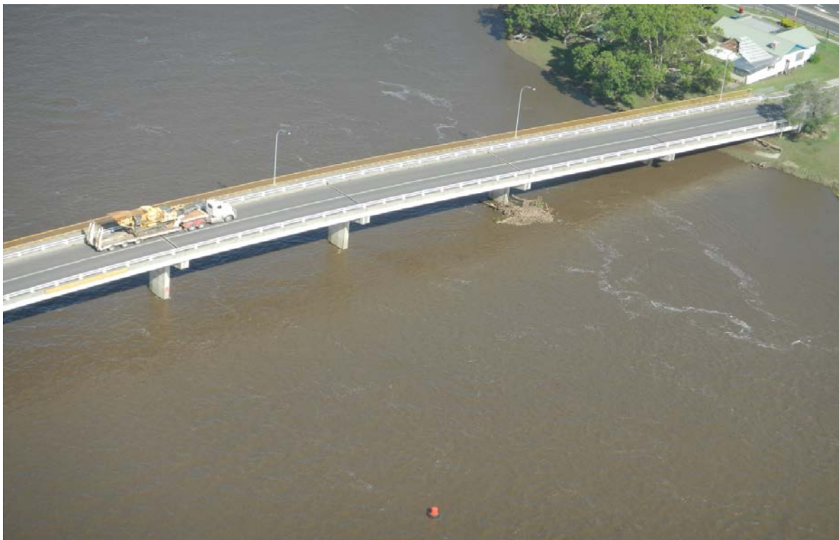
Plate C -10 Richmond River (Woodburn Bridge) (1 February 2013, 3.24pm), showing minor evidence of debris blockage around bridge piers.
