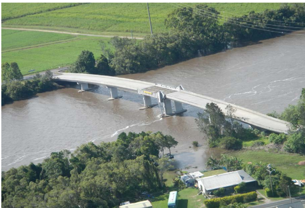
Plate C -11 Richmond River (Broadwater Bridge) (1 February 2013, 3.29pm), showing no evidence of debris blockage.
