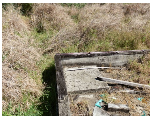
Figure E-19: Close up of south-west corner of concrete slab, low walls and timber top.
