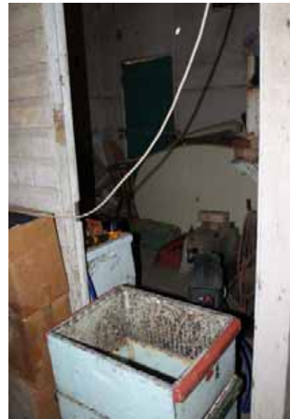
Figure 7-103: Interior of enclosed barn section of dairy, facing south-east, photo taken by Rachael Loizou on 31 October 2011.
