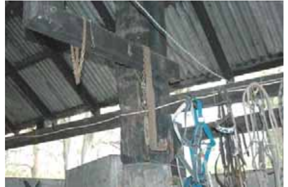
Figure 7-94: Hand forged iron hooks which have been removed, facing south-west (Heritage Concepts 2007).
