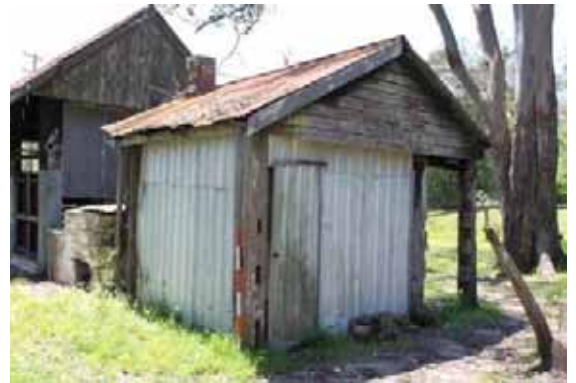
Figure 7-96: Structure to south of main structure, facing north-east, photo taken by Rachael Loizou on 25 October 2011.
