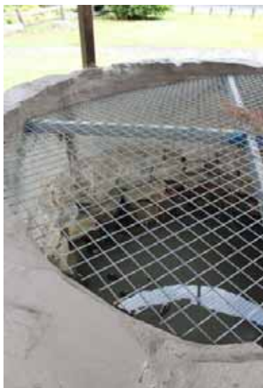
Figure 7-73: Interior to stone-lined well with metal mesh cover and rendered and painted concrete capping, facing north-north-west, photo taken by Rachael Loizou on 26 October 2011.
