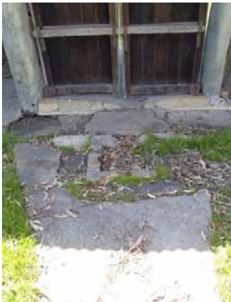
Figure 7-91: Discharge drain to west of main structure, facing east, photo taken by Rachael Loizou on 25 October 2011.
