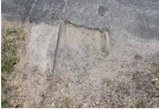
Figure 7-51: Petticoat Lane Tram Tracks, facing west, photo taken by Rachael Loizou on 31 October 2011.
